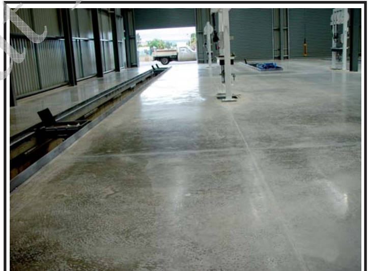
Caopower South Australia used Densi-Proof plus Surface Sheen at time of pour and virtually eliminated any cracking. They have a hardened surface that protects against oil, acid attack, and is attractive and easy to clean.
