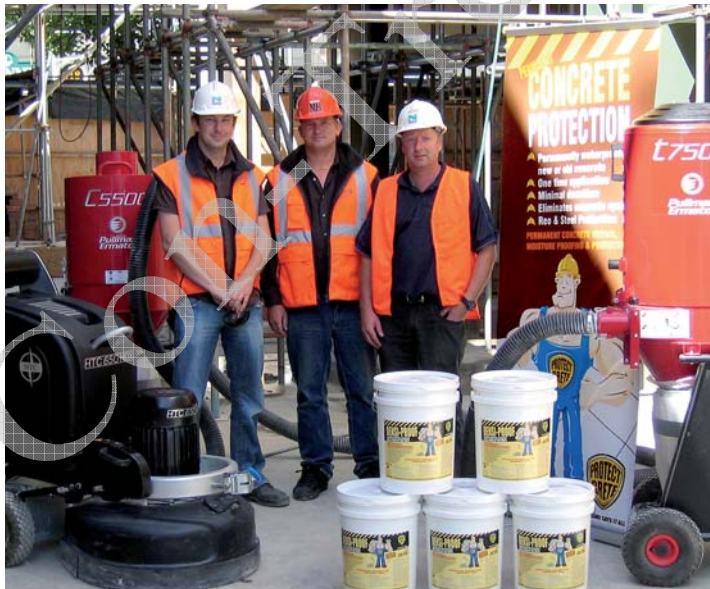
Left to right. Blair McGill , Naylor Love Project Manager, Barrie Clydesdale , Mulford Holdings Densi-Proof trained applicator and Craig Kennelly , Gilt Edge Industries Regional Manager – Protect Crete distributor on site at the start of stage 1.
